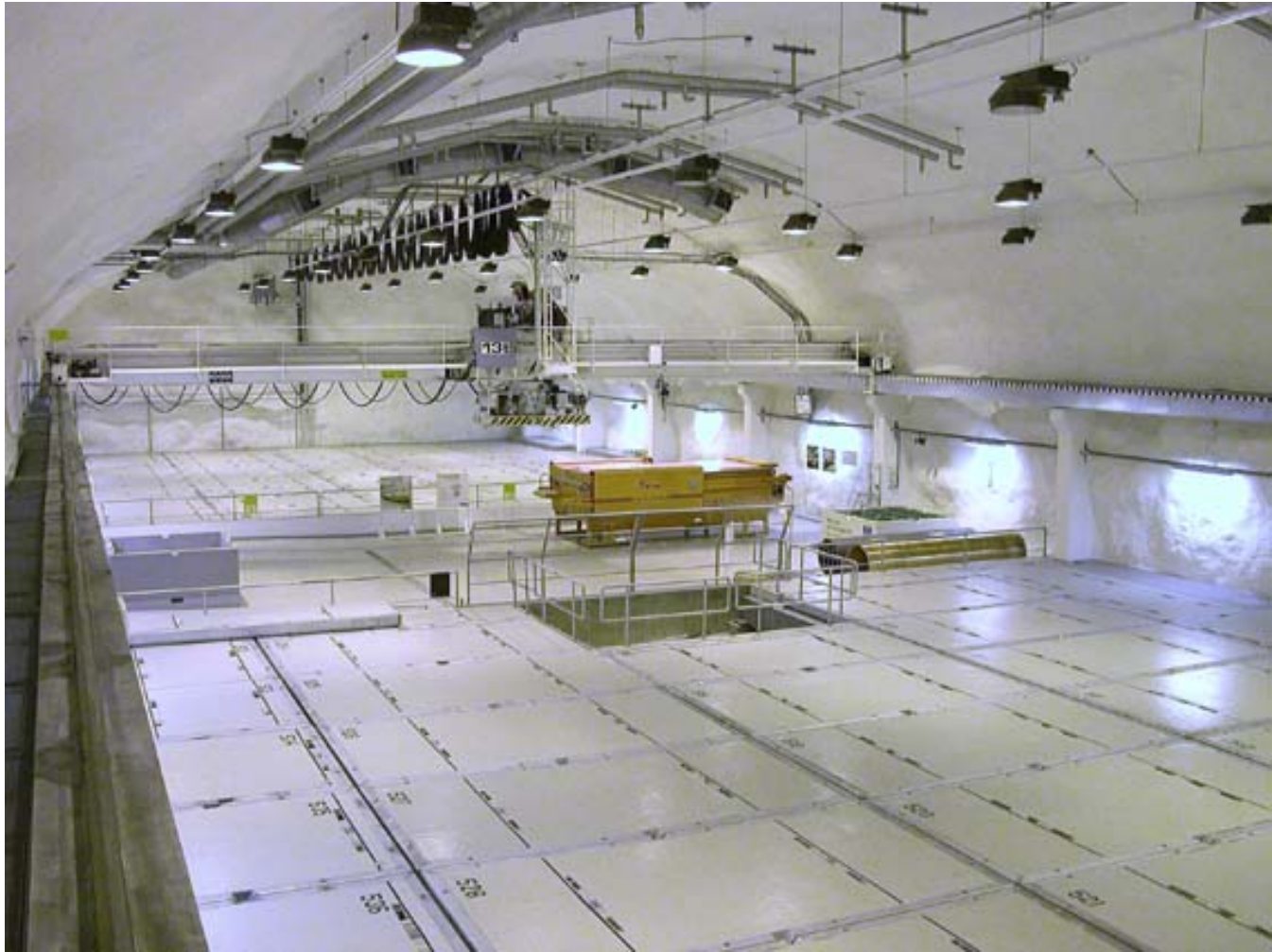
Low-level and intermediate-level waste repository at Olkiluoto in Finland (Posiva)
